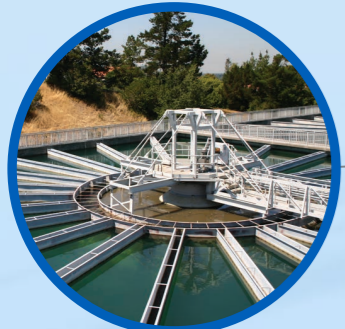
Rinconada Water Treatment Plant
