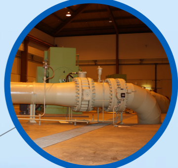
Coyote Pump Plant
