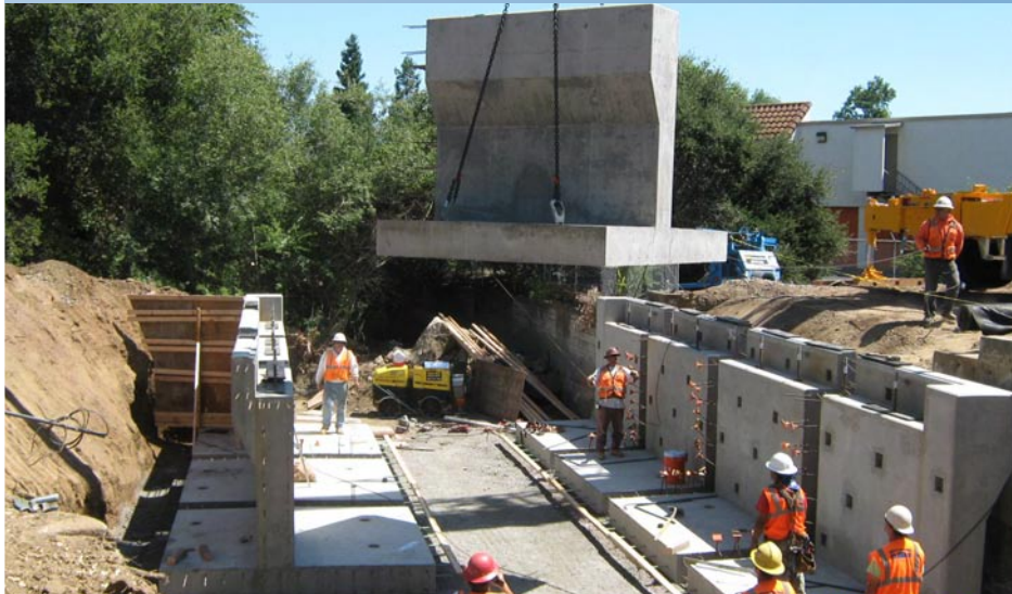
Calabazas Creek Flood Protection Project kicked off its second construction season this summer with the demolition and widening of the Union Pacific Railroad (UPRR) bridge. Crews removed the old bridge and replaced it with a wider culvert underneath the railroad bridge. Photo taken July 27, 2011.
