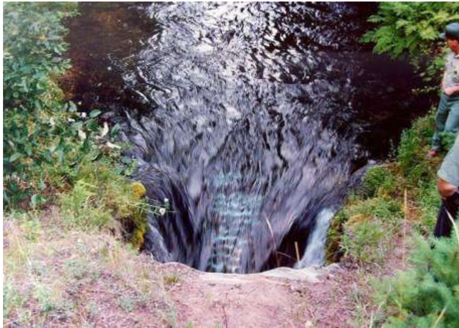
Figure 6-2. Excessive Flow Velocity Downstream of a Culvert (From US Dept of Agriculture Forestry Dept.)
