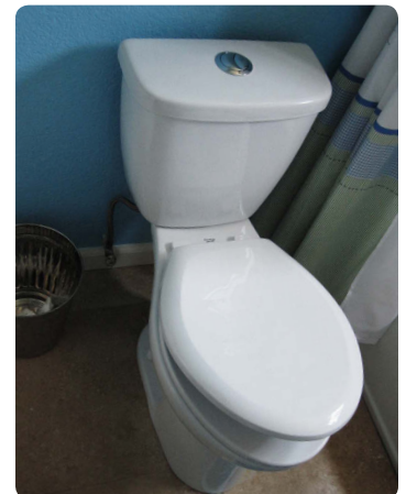
High efficiency toilet.
