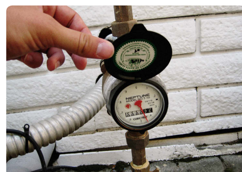
Residential water submeter.
