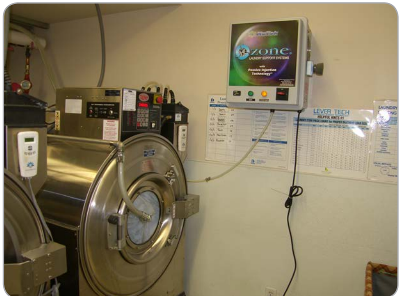
Ozone laundry system at hotel, a WET Rebate Program participant
