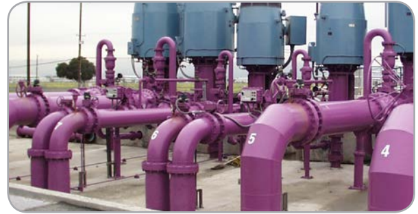
Recycled water pumps
