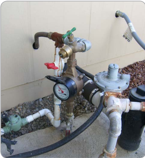
Water submeter installed at a mobile home park in San Jose
