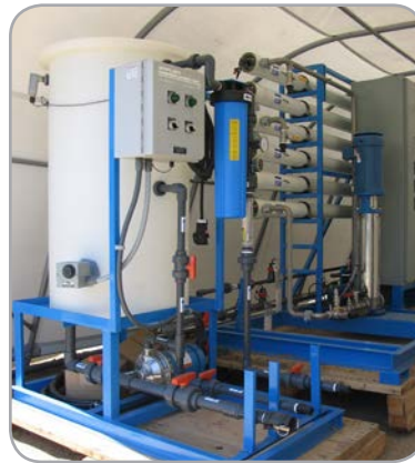
RO desalination pilot
