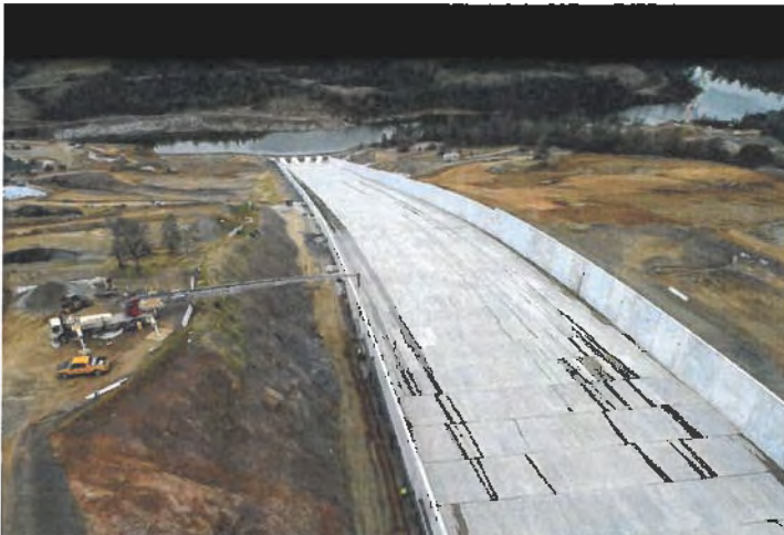
A view of the recently completed Lake Oroville main spillway. Backfill operations continue to raise the area around the underdrain piping system outside the sidewalls of the spillway. DWR/2019
