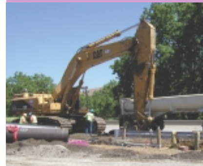
The Silver Creek pipeline, currently in construction, will deliver recycled water to the Metcalf Energy Center, a new Calpine power plant being built in Coyote Valley.
