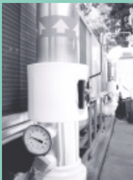
A Water Efficient Technology (WET) Program rebate will go to this air-cooled chiller retrofit project at Palo Alto Unified School District.
