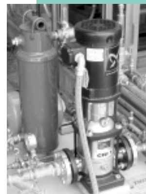
Stanford University’s closed loop cooling system has been projected to save over seven million gallons of water annually.
