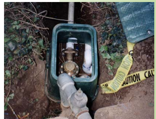
The District is conducting two pilot programs to see if the installation of submeters like this one reduce water usage.
