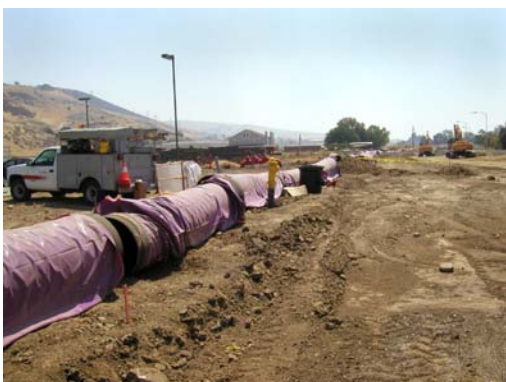
The Silver Creek pipeline extension will deliver recycled water to the Metcalf Energy Center, a new Calpine power plant being built in Coyote Valley.
