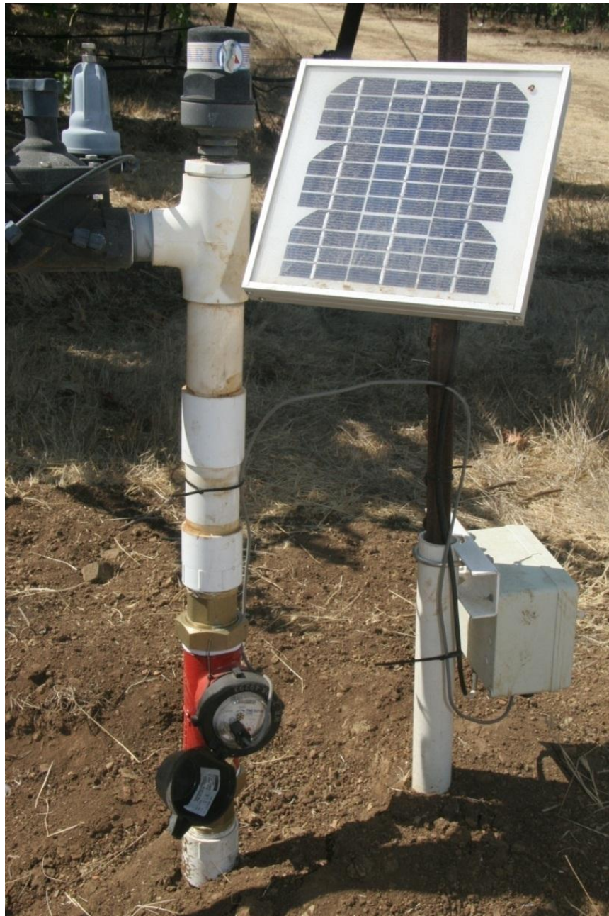
flow monitoring data logging array
