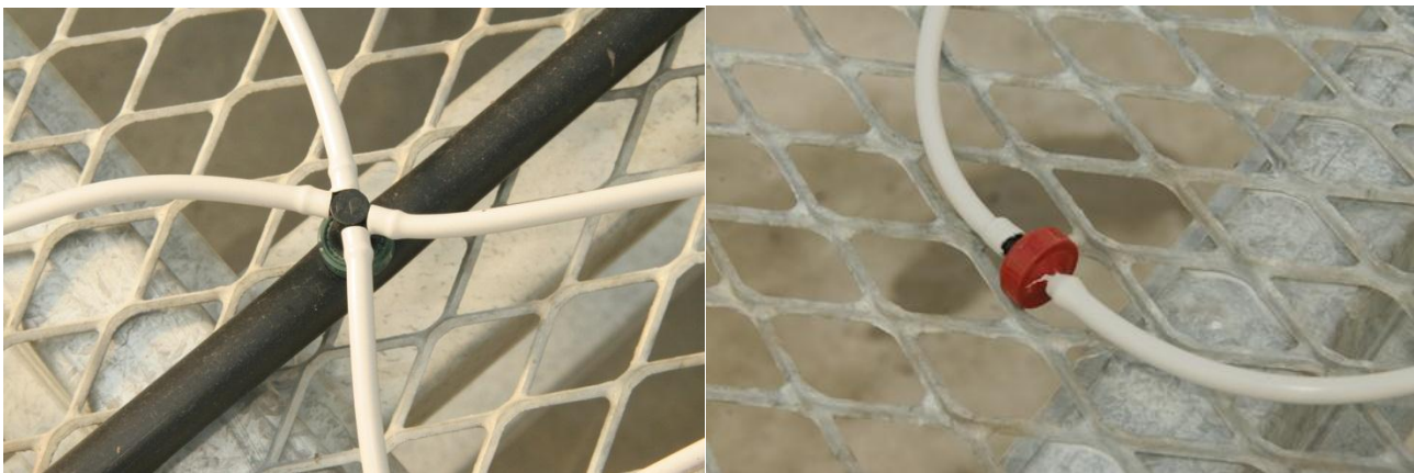
4-way split of emitter tubing from pressure-compensating emitter off submain (each line runs to a single pot or is pinched off if/when pots are removed; pressure compensating emitter installed in-line during test.)
