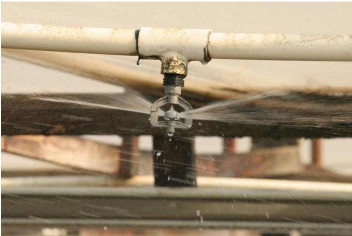
Existing sprinklers (above) and rotators (below)
