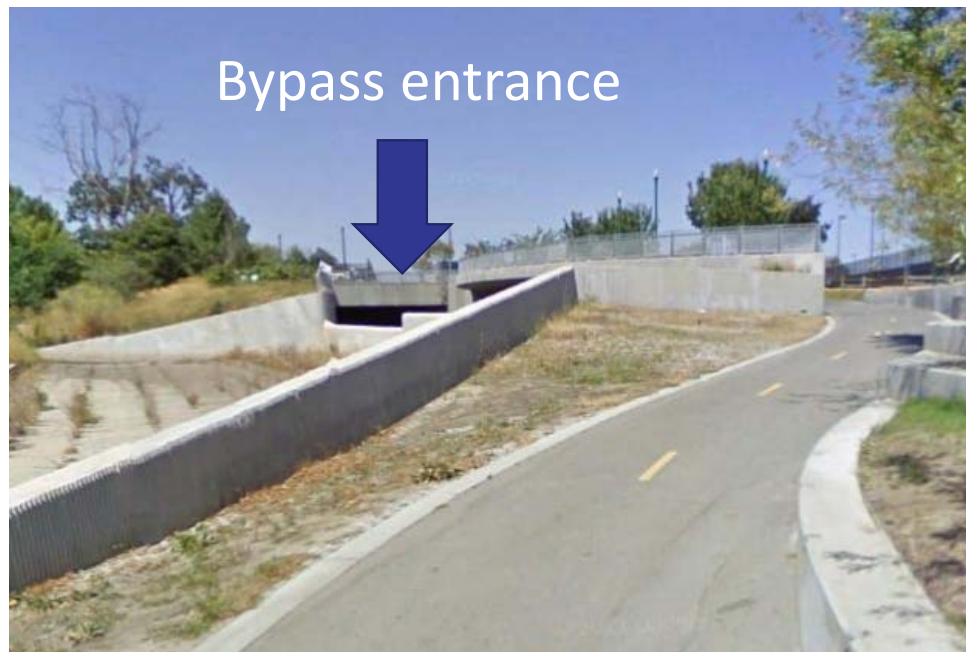
Bypass Culvert Concrete pipe that diverts water
