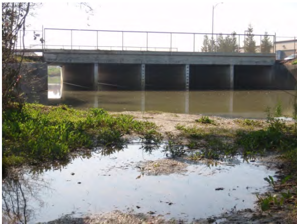
Figure 2-12. Lower Silver Creek looking at the downstream face of the Tully Road Bridge
