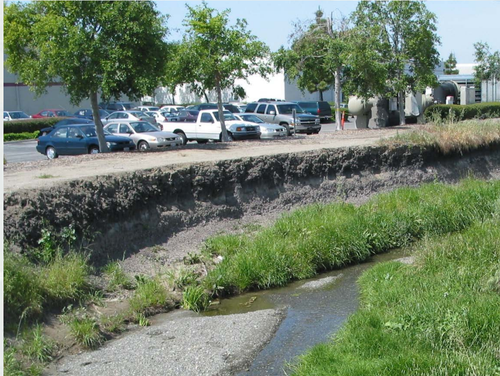
Berryessa Creek Bank Erosion
